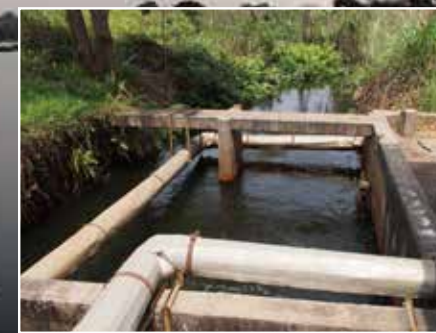
THE IRRIGATION system in M'bé has degraded due to wear and tear.
